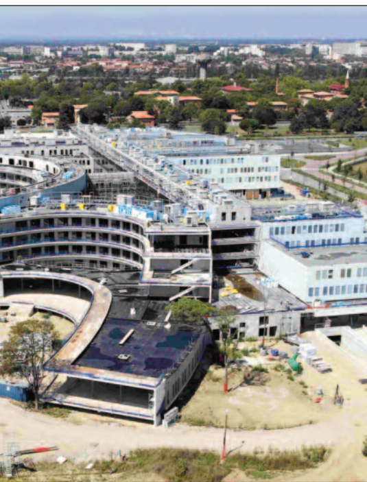
Like a phoenix from the ashes. The Toulouse oncopole is built on land left devastated by a catastrophic explosion at a chemical works in 2001. The University Cancer Hospital – the curved building in the centre – will open in early 2013
